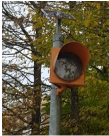
2. Traffic Light with solar panel at Gököy Campus (BAİBU, Turkey)
