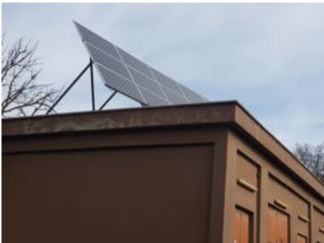
3. Roof Mounted Solar Panels at Gököy Campus (BAİBU, Turkey)
