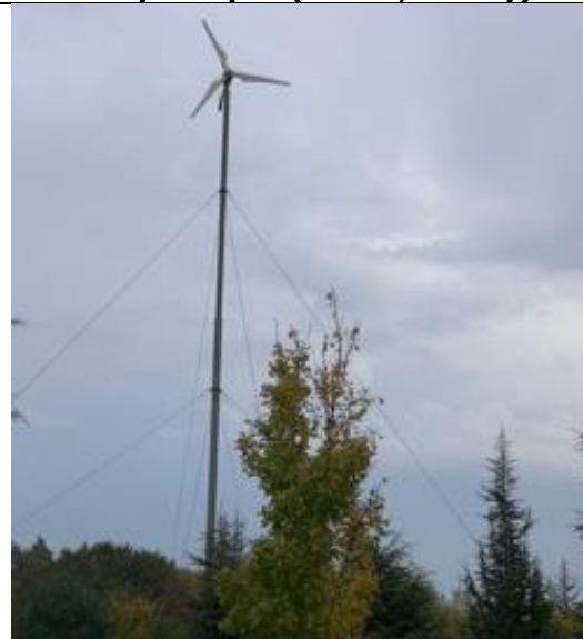
4. Wind Turbine at Gököy Campus (BAİBU, Turkey)
