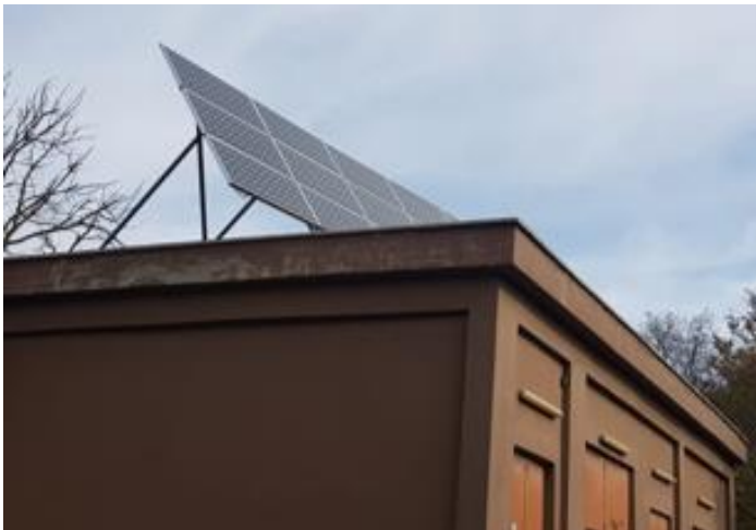
3. Roof Mounted Solar Panels at Gököy Campus (BAIBU, Turkey)
