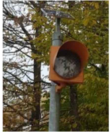
2. Traffic Light with Solar Panel at Gölköy Campus (BAIBU, Türkiye)
