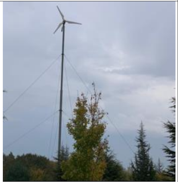
4. Wind Turbine at Gölköy Campus (BAIBU, Türkiye)
