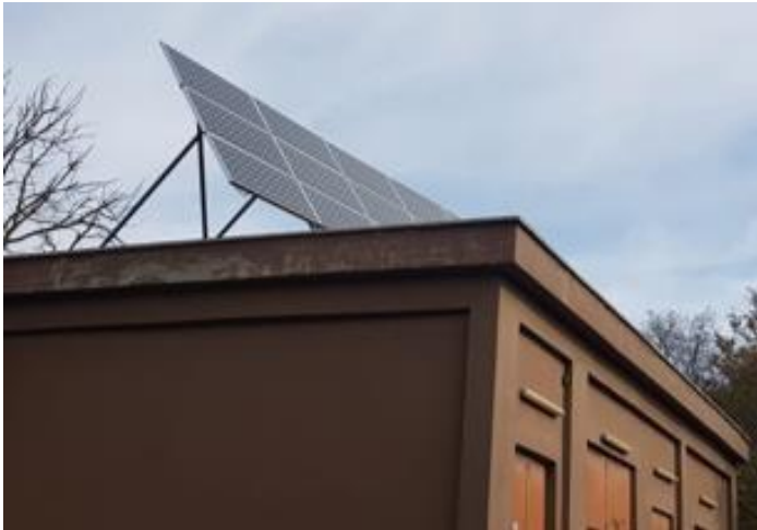
3. Roof Mounted Solar Panels at Gölköy Campus (BAIBU, Türkiye)
