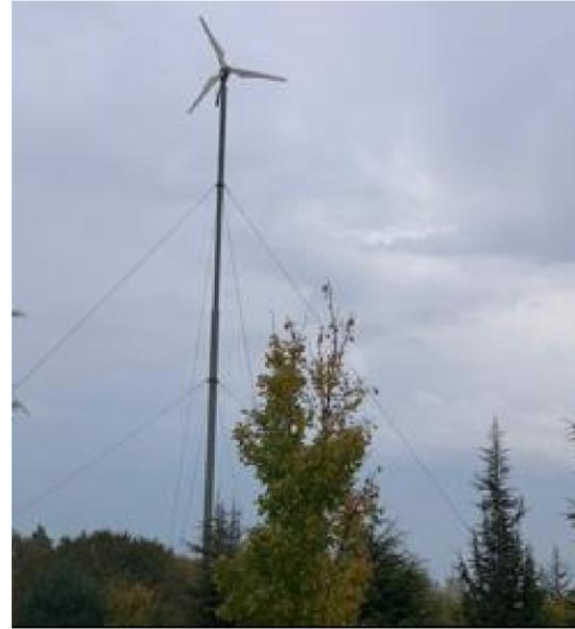
4. Wind Turbine at Gököy Campus (BAIBU, Türkiye)
